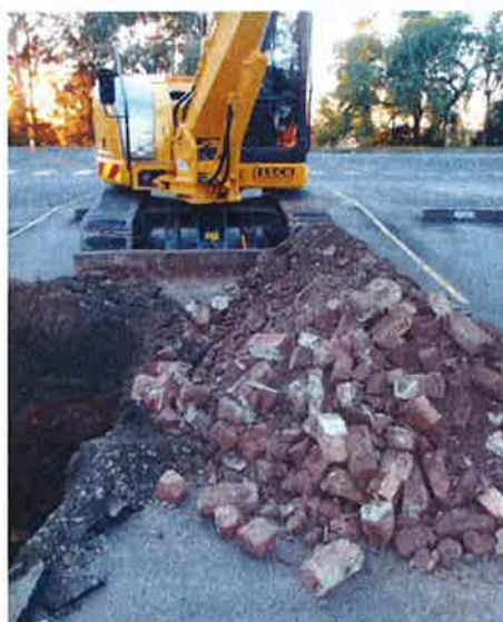
Photo 3 – Rubble at TP40
